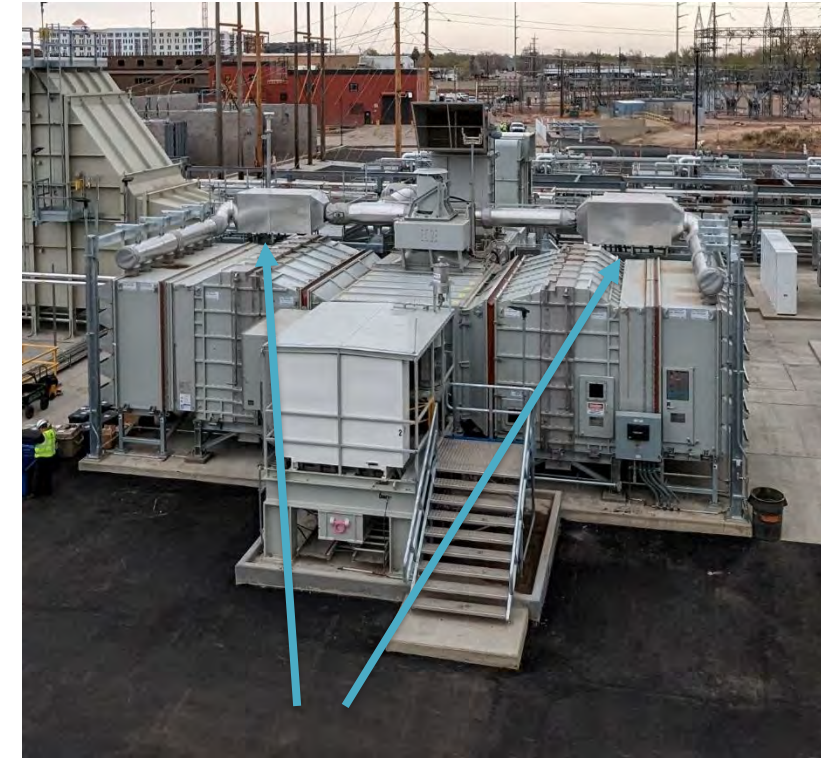
Electric Heaters and Air Injection
