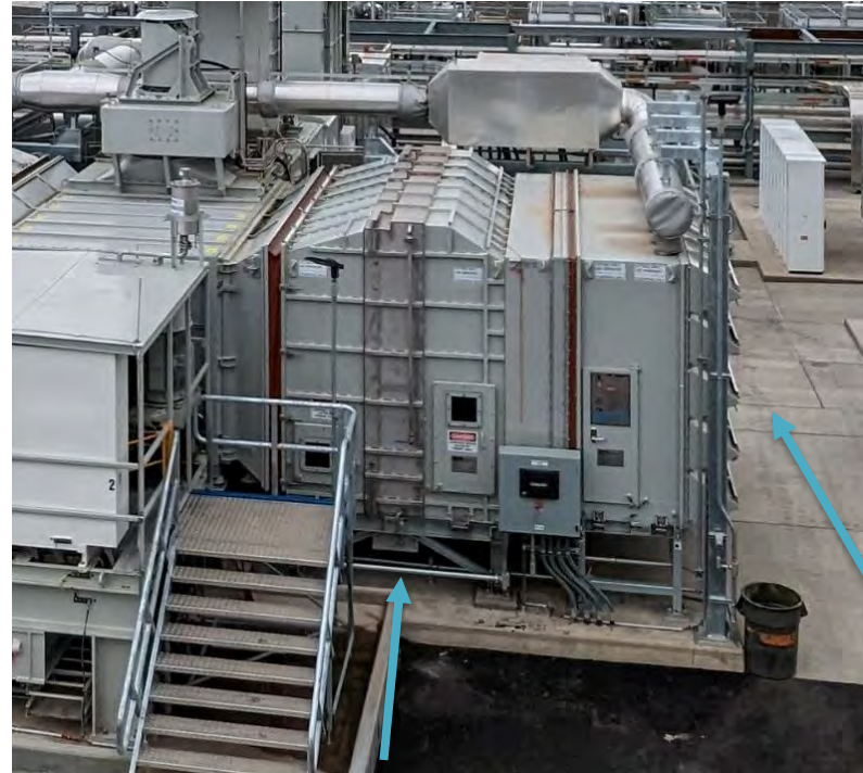
Water Spray Module w/ Drift Eliminator
