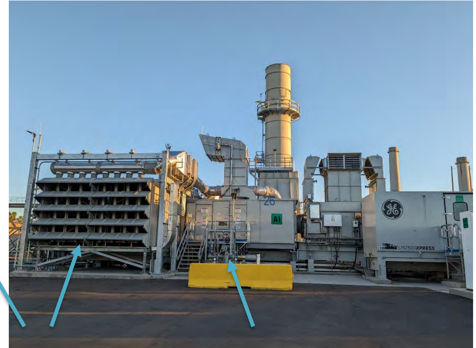
Gas Turbine Air Inlet
