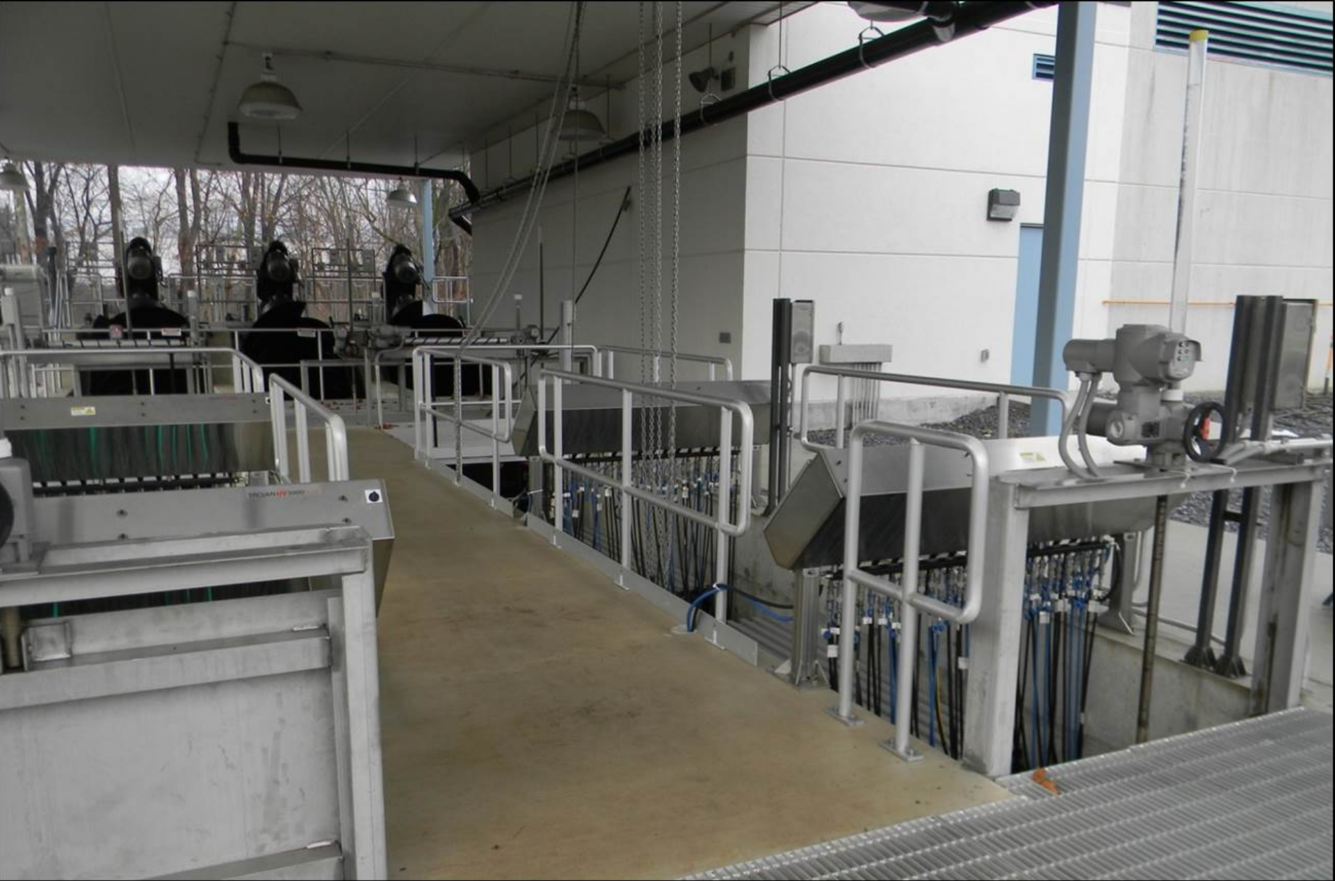
Ultraviolet Disinfection System
