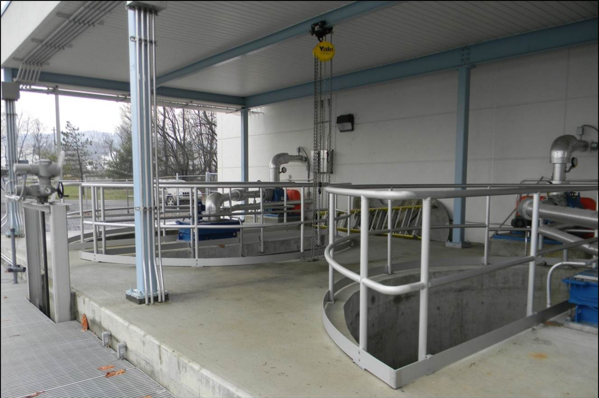
Vortex Grit Separation System (preserve influent carbon)
