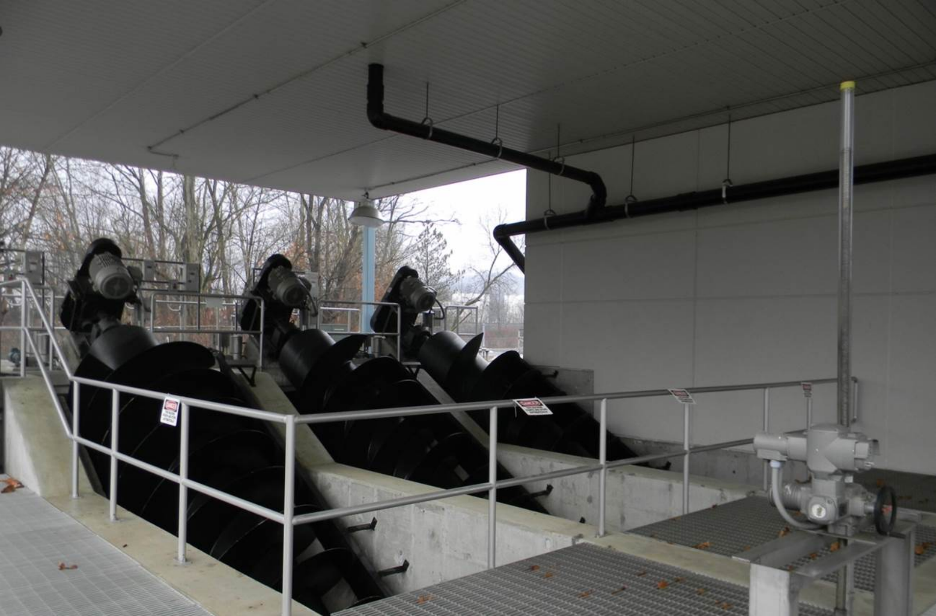
60" Diameter Screw Lift Flood Pumps
