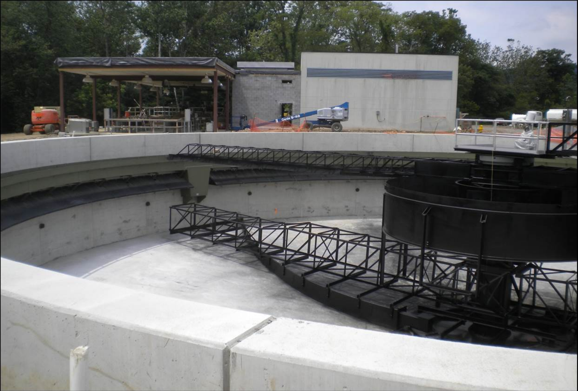
Final Clarifiers with Stamford Baffles
