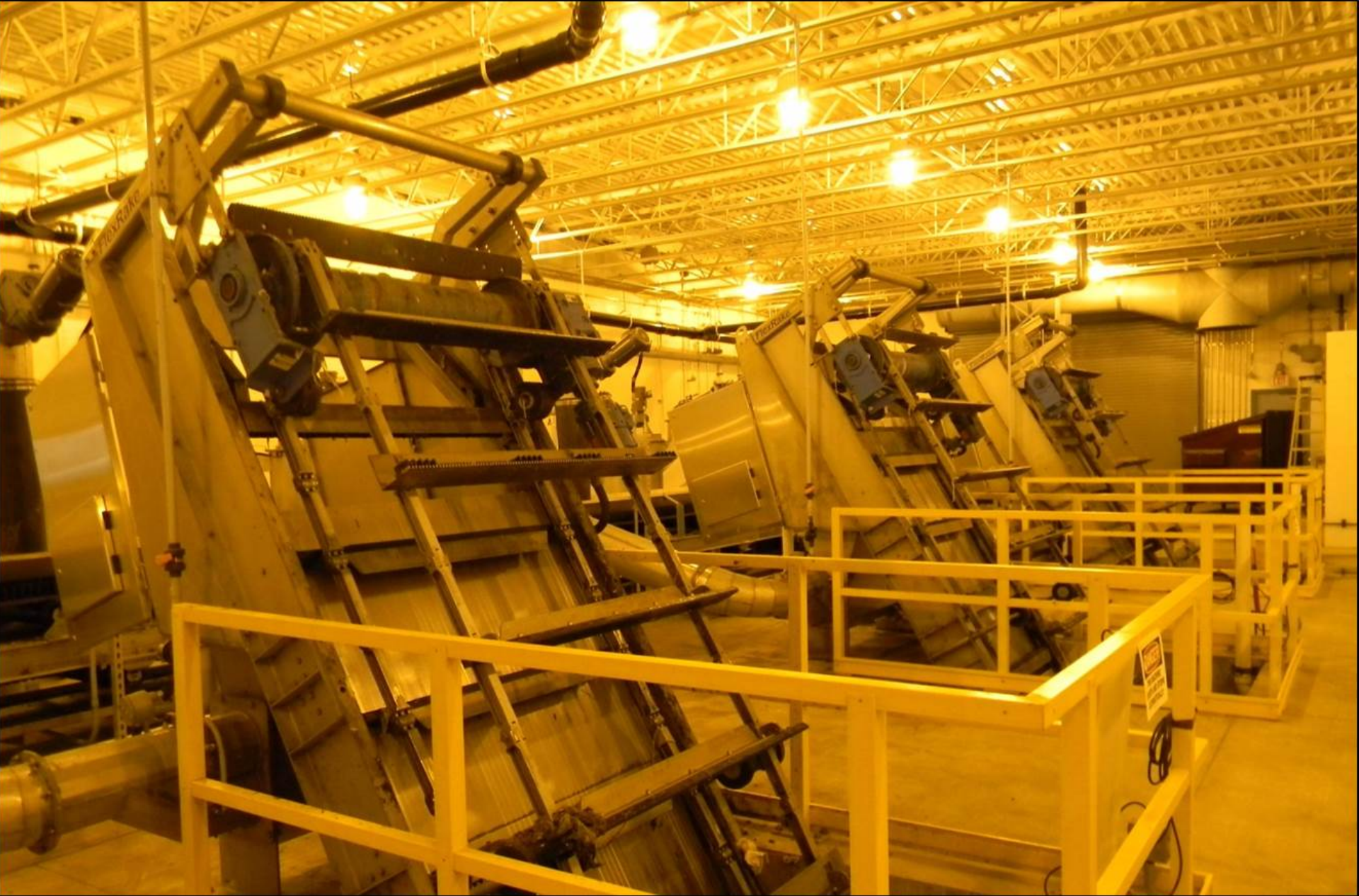
Headworks Fine Screening
