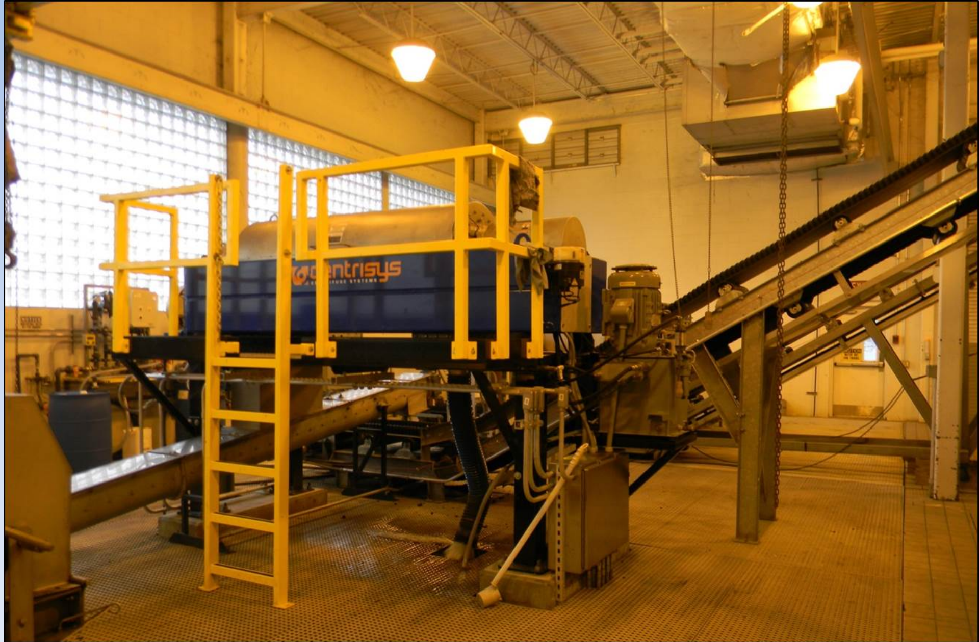
Centrifuge Sludge Dewatering System
