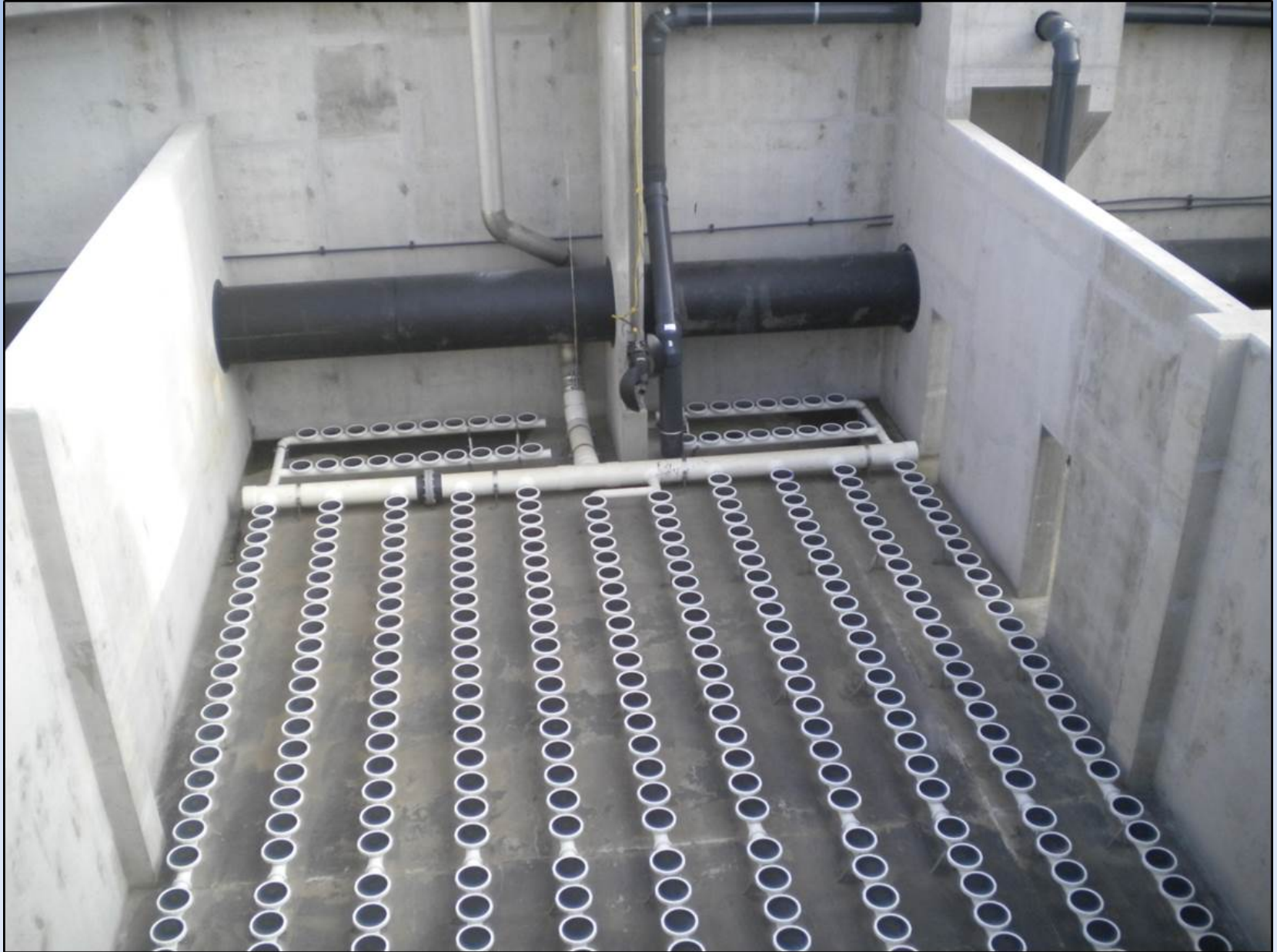
Switch Zone – Membrane Diffusers (oxic) & Submersible Mixers (anoxic)
