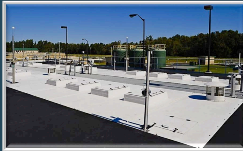
MBT Tanks w/Covers
