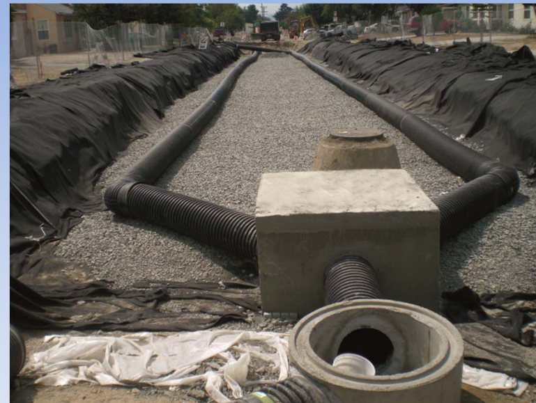
Elmer Avenue Infiltration Gallery
