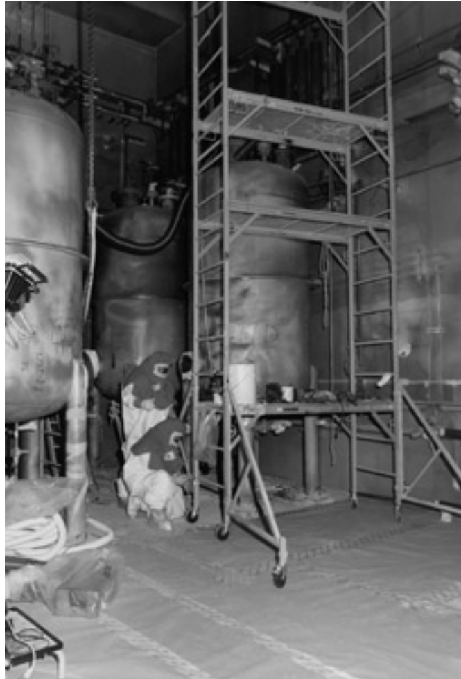
Areas in former plutonium processing facilities at Rocky Flats contained extremely high levels of contamination. Some areas were known as “infinity rooms” because radiation levels pegged measurement equipment used at Rocky Flats 20 years ago.
