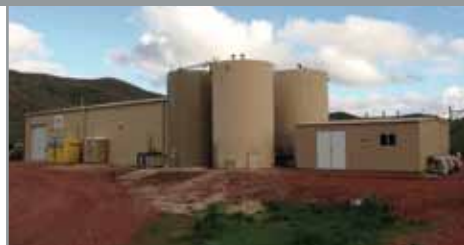
Marathon Oil Company sought a reliable water treatment process for their Sheridan, Wyoming gas field. Through design-build delivery, CDM Smith implemented a first-of-its-kind, innovative water treatment and reuse system that meets water discharge limits, protects fresh water supplies and controls treatment costs for Marathon.
