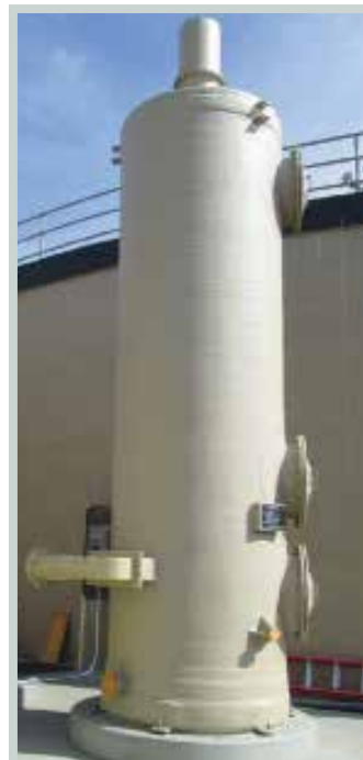
Finished Biotrickling filter system.
