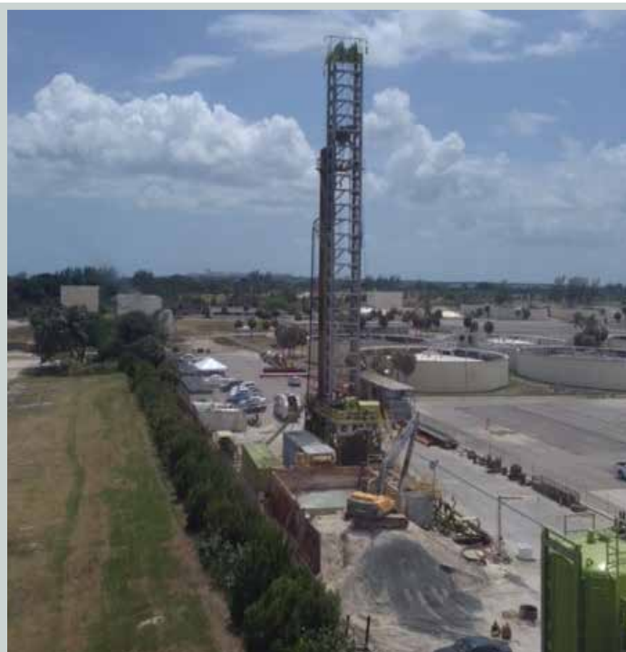
The success of the OOL Program relies on an alternative disposal method: deep injection wells capable of receiving more than 15 mgd of treated wastewater each.
